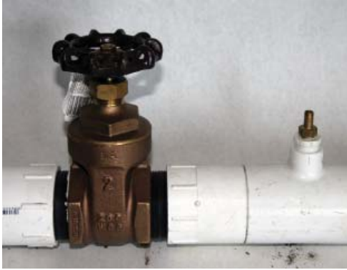
Figure 1. A gate valve with a Schrader valve allows pressure to be adjusted and monitored in an irrigation block, but the valve must be adjusted manually to compensate for changes in upstream pressure.
